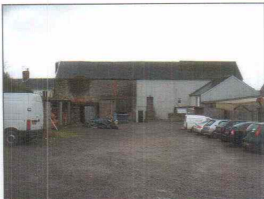
Rear of Wool Store with rough surfaced car park and yard. No ground level access to the building available
